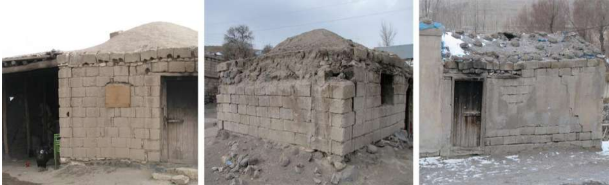
Figure 3. Observed damage due to use of heavy earthen roofs
