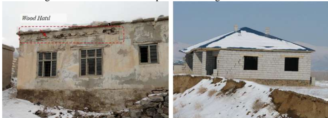
Figure 4. Damage due to lack of hatil systems
