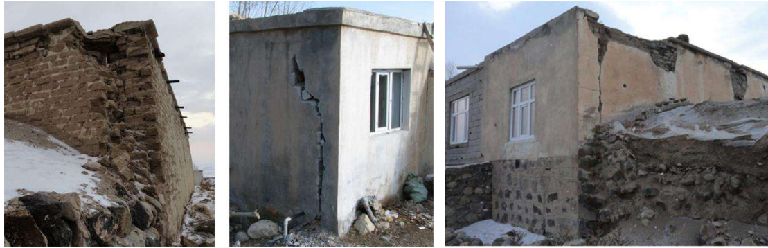
Figure 5. Observed corner damage
