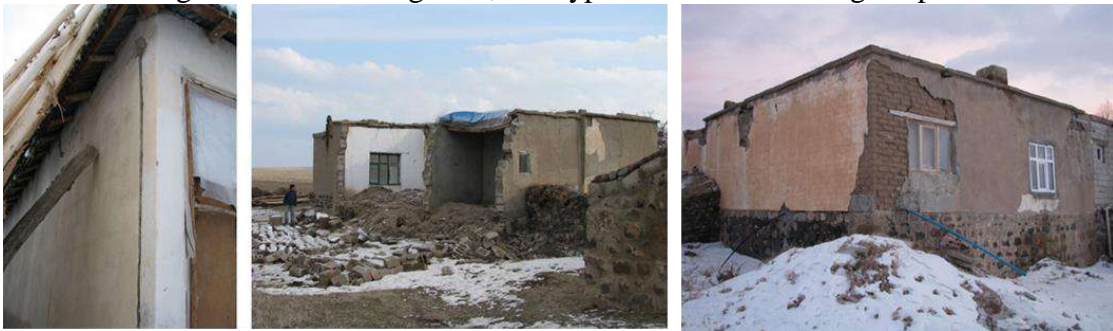
Figure 6. Observed damage due to separation of walls and the plaster effect
