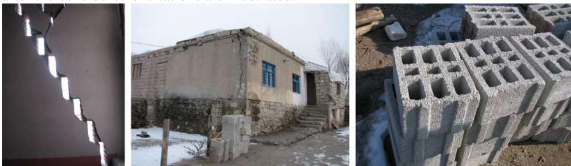
Figure 2. Damage due to use of HCT
