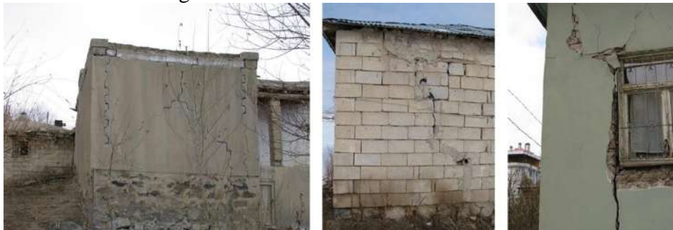
Figure 7. Observed in-plane damage
