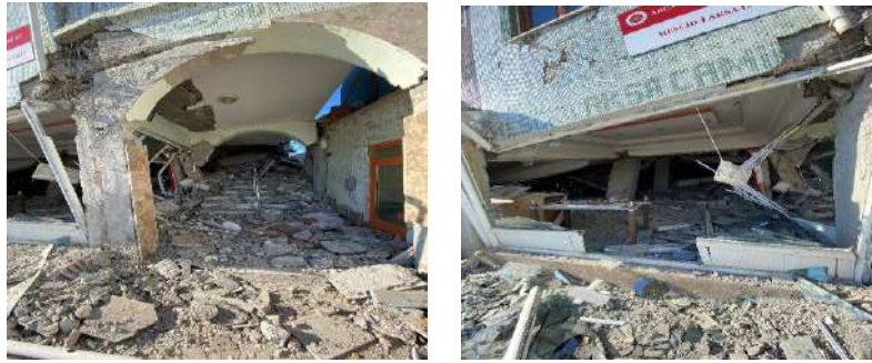
Figure 7. Examples of damage due to soft storey [9]
