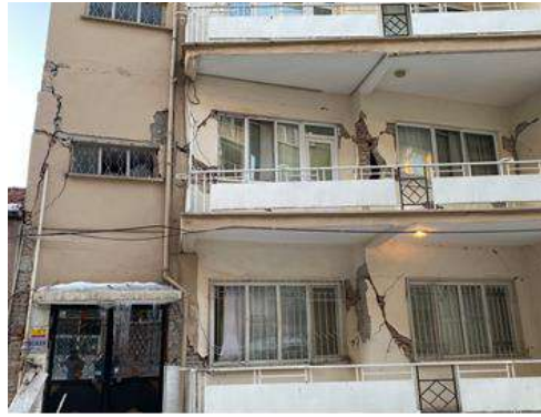
Figure 14. A masonry structure with a corner failure mechanism and shear cracks (38.35371 N, 38.32353 E) [17]
