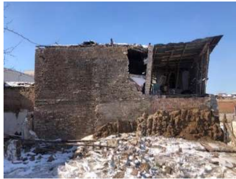
Figure 15. Damage distribution of a masonry structure (38.35267 N, 38.31155 E) [17]
