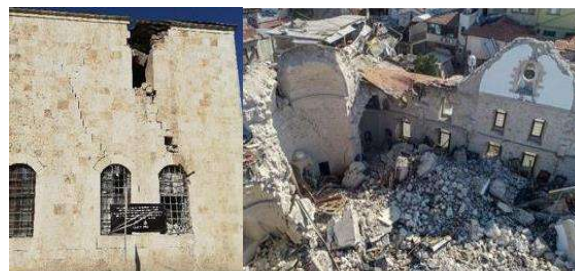
Figure 13. Damaged historical structures in Antakya after earthquake sequence; a) Habib-i Neccar Mosque (courtesy of the EEAT), b) Rum Orthodox Church [19]
