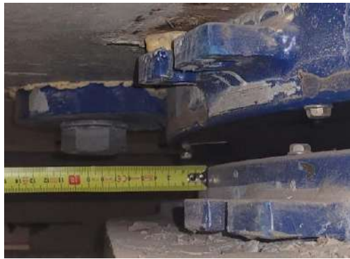
Figure 10. Residual isolator displacement in Osmaniye State Hospital [12]
