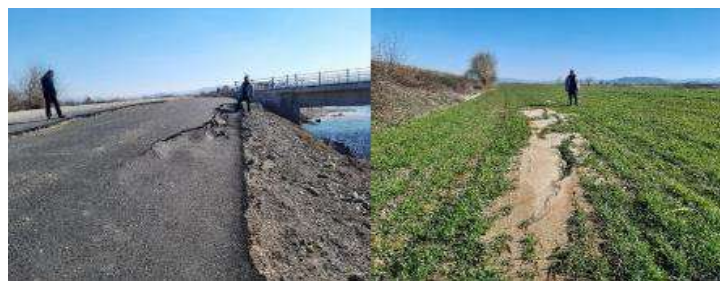
Figure 11. a) Lateral spreading (left), b) sand boiling due to soil liquefaction (right) [19]
