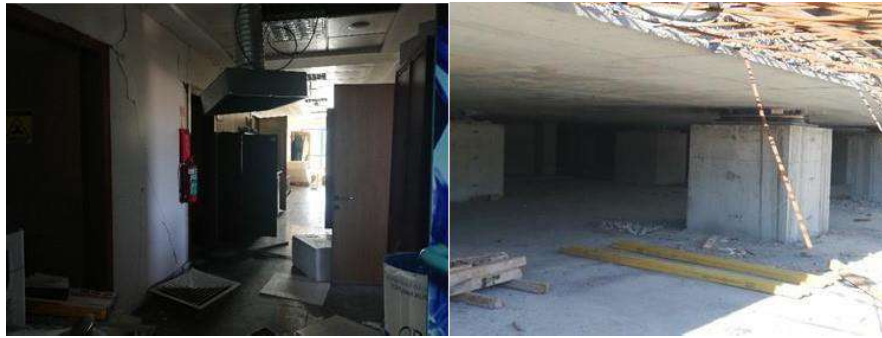
Figure 17. a) Existing city hospital in Kahramanmaraş with extensive non-structural damage, b) a new hospital construction in Kahramanmaraş with base isolation system (the isolators worked and performed well during the earthquake although most of them were not installed yet) (courtesy of the EEAT) [19]
