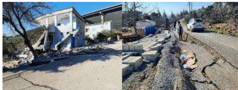
Figure 7. a) Major damage to houses due to surface faulting (left), b) deformations and settlements due to surface faulting on the road in Nurdagi (right) [19]
