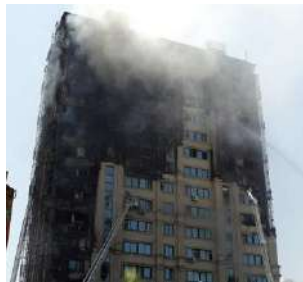
Figure 1. Facade system with a ventilated air gap of a residential building after a fire, Baku, next to Azadlig metro station, 2015 [5]
