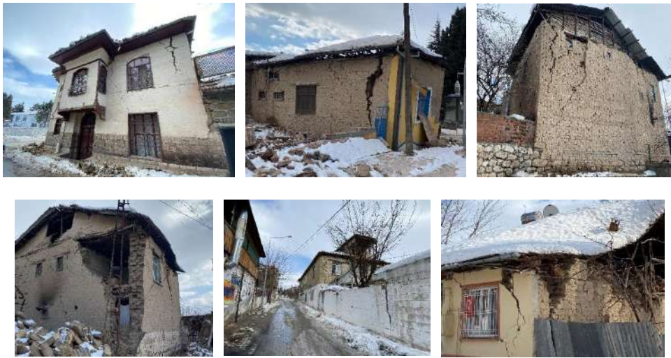
Figure 18. Corner failure mechanisms in masonry structures in Gündüzbey district [17]
