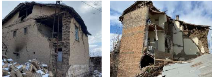
Figure 14. Failures caused by out-of-plane movement in masonry structures in Malatya [10]
