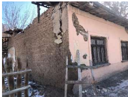
Figure 16. Damage distribution in a single storey masonry building (38.35256 N, 38.31163 E) [17]
