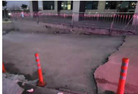
Figure 6. The access ramps of the hospital building cracked and deformed in places where the seismic gap would have been [11]
