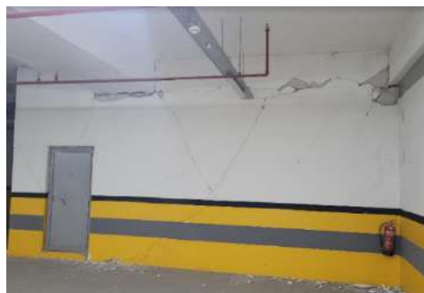
Figure 5. Infill walls at the isolator (parking) story, constraining the movement of the isolated superstructure [10]
