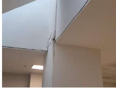
Figure 1. Cracking and slight damage in gypsum boards covering the seismic isolators due to displacement during the earthquakes [10]
