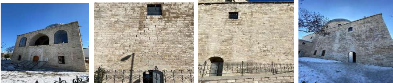
Figure 9. Damage distribution of Taşhoran Culture and Art Center [10]
