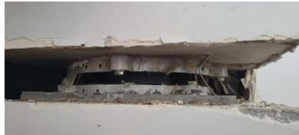
Figure 2. One of the friction pendulum type seismic isolators of Elbistan State Hospital [10]
