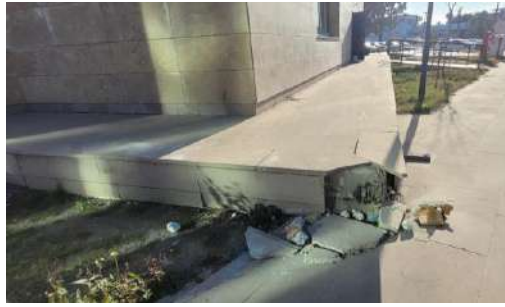
Figure 9. Minor collision damage between a corner of the isolated structure and the pavement [11]
