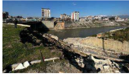
Figure 9. Settlements in alluvial soils along the Asi River in Hatay and damage to retaining walls due to lateral spreading [19]
