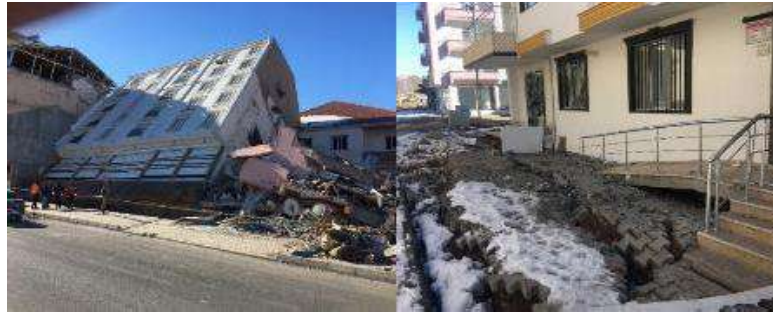
Figure 6. Tilting of buildings and heaving of soils around foundations due to liq-uefaction (Adiyaman- Golbasi) [19]
