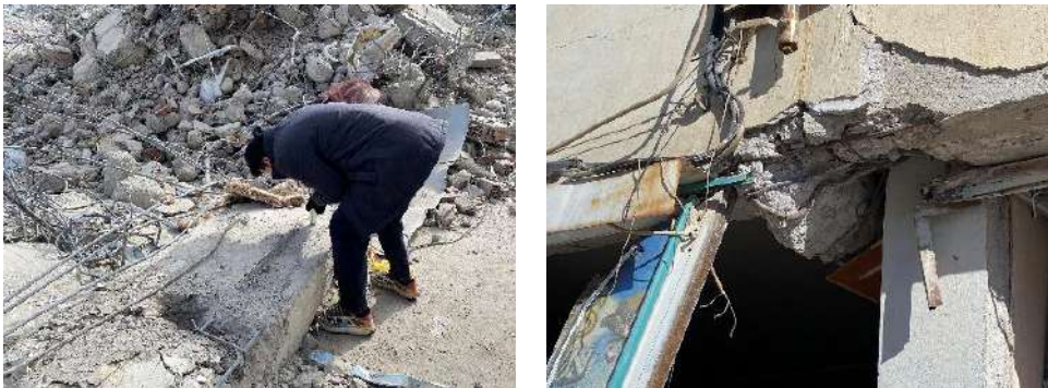
Figure 13. Poor quality of materials [10]
