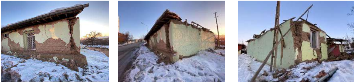
Figure 17. A masonry structure that combines the causes of the corner collapse mechanism (38.31279 N, 38.25054 E) [17]
