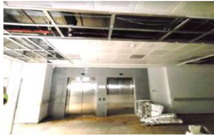
Figure 12. Flood damage at upper stories of isolated superstructure and resulting red (rust) residue at Osmaniye State Hospital [12]
